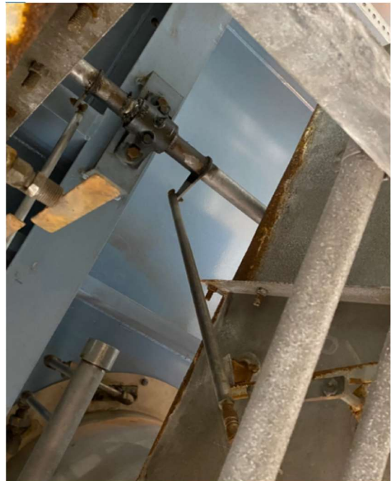
Figure 4: Fired Heater burner with jackshaft rod connection to actuator drive shaft shown.
