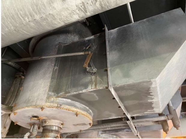
Figure 3: Fired Heater burner with jackshaft lever rod connection to burner register assembly shown.
