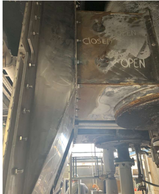
Figure 6: Birwelco USA Burner Compensator fit up to existing burners.
