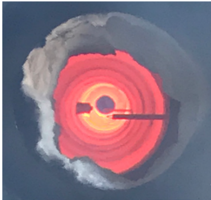
Figure 3 – View through sight glass at base of stack looking back towards the burner
