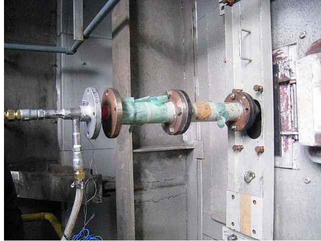
Figure 4. Photo of the ash deposition test probe inserted in boiler.
